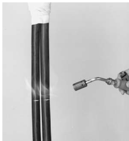
6. Flame-brush the cables over the cleaned and abraded areas for about 10 seconds.
