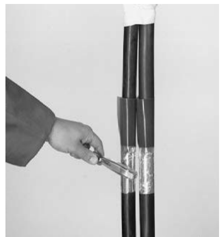
8. Dress the aluminium of the cable wrap down with a blunt tool to smooth sharp edges.
